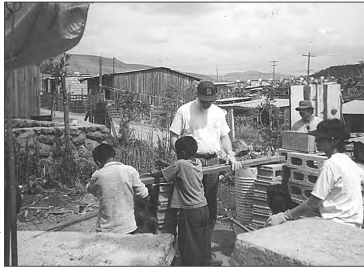
Two Honduran boys help Franciscan Father Martin Day, center, measure a board to be used in the construction of a new home. Carlos Montanez, back, and Gina St. Hilaire, front, look on. Father Day, pastor of St. Joseph Parish in Terre Haute, and 14 parishioners traveled to Honduras last month to help build homes and to deliver medicine.
